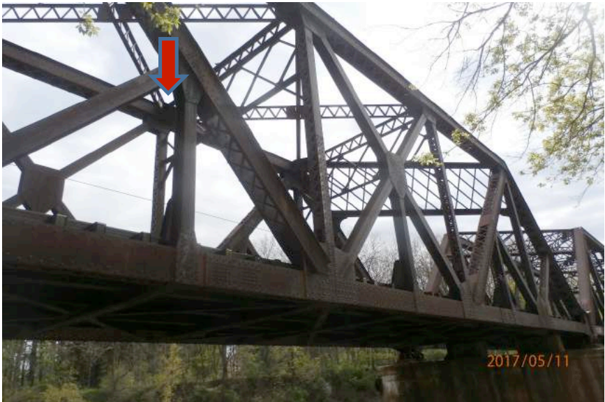
Figure 4: Railroad bridge over the Erie Canal in Pittsford, NY. Photo courtesy of Sarah Piecuch, NYSDOT.
